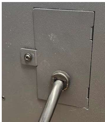
Figure 2: Existing Power Cord Strain Relief
